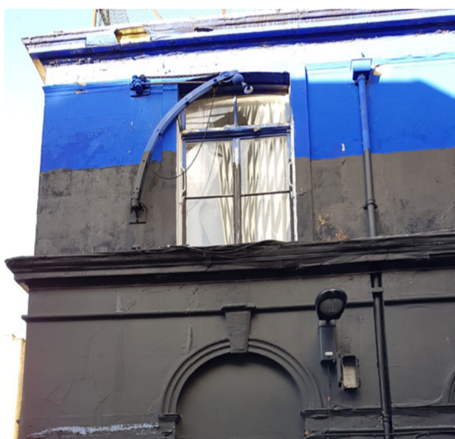
Existing wall crane
